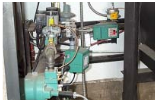
Valve Train and Burner
